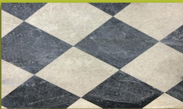
BEFORE – Senior Living Facility (Floors in the laundry room which is a heavy traffic area)
