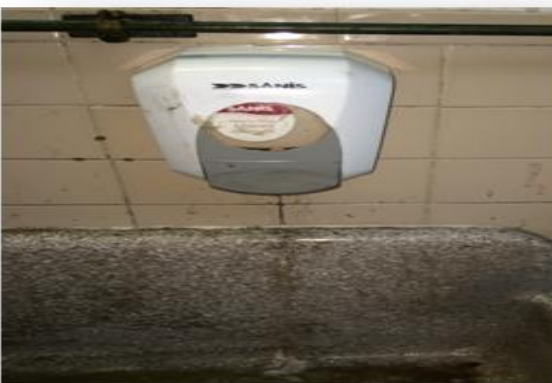
BEFORE –Service Restroom Soap Dispenser Area
