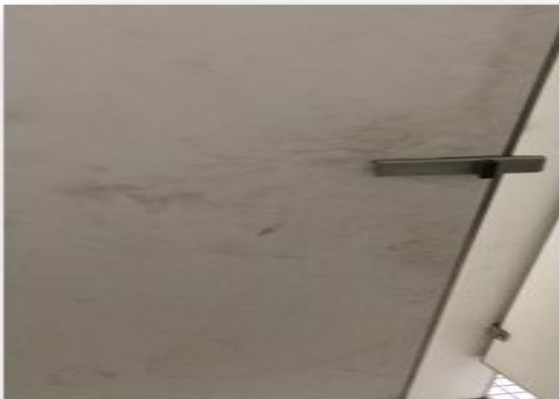
BEFORE –Service Restroom Stall Door
