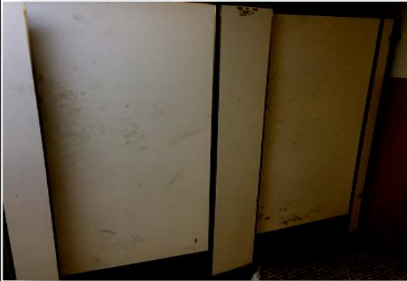
BEFORE –Service Restroom Stall Door
