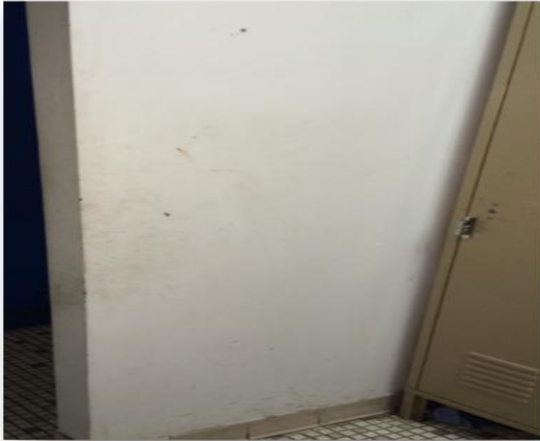
BEFORE – Service Area Restroom Walls
